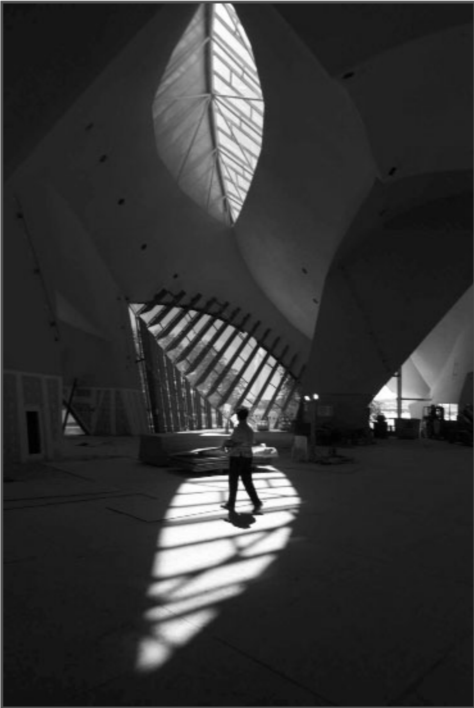
Dawn Casey walks through the Main Hall of the National Museum of Australia during its construction. Photo: Fairfax.
